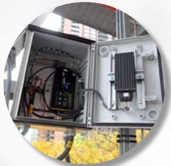
1. Directional antennas of the DATAEAGLE Classic 3702A master at the control cabinet at a mast.
