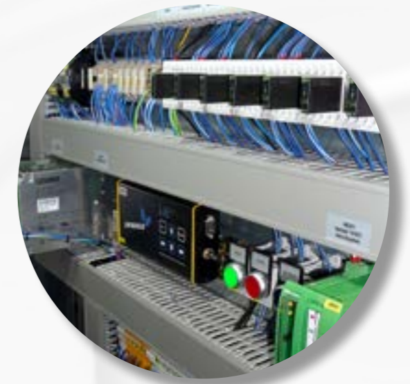
2. Up to now, DATAEAGLE 3000 Master in the control cabinet has been communicating reliably with the cabin.
