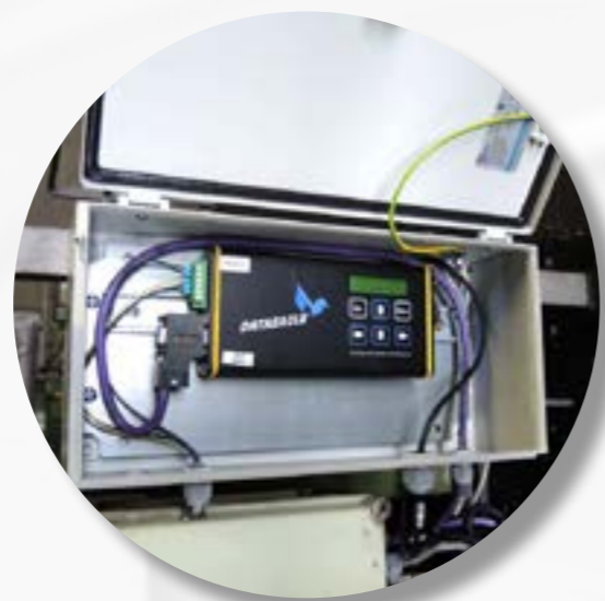
2. DATAEAGLE Classic 3000 applied at Pfänder tunnel.
