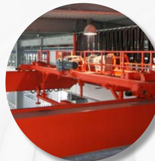
1. The crane trolley in the galvanizing plant receives and sends data via DATAEAGLE slave.
