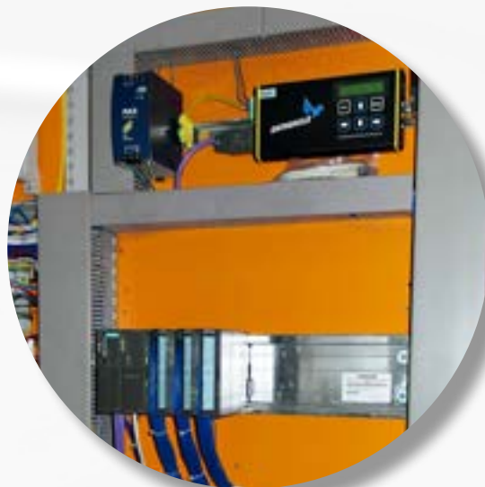
2. DATAEAGLE Master in the control cabinet directly at the clarification tank.
