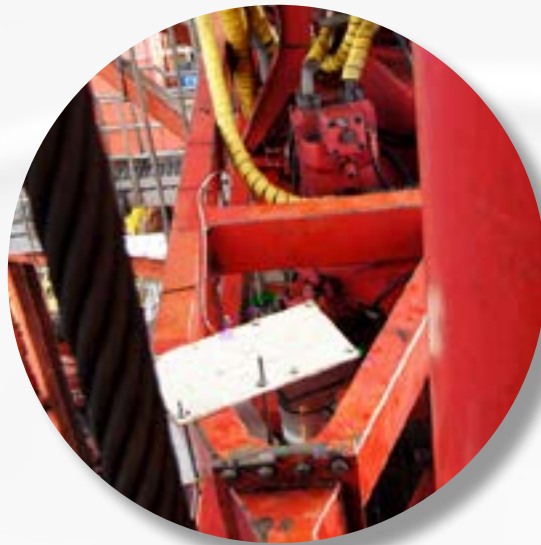
2. DATAEAGLE at the mobile side of the plant by which the drill pipe is installed.
