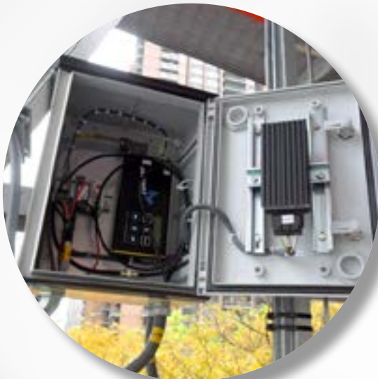
1. Directional antennas of the DATAEAGLE Classic 3702A master at the control cabinet at a mast.
