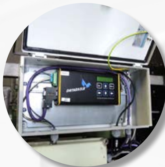
2. DATAEAGLE Classic 3000 applied at Pfänder tunnel.
