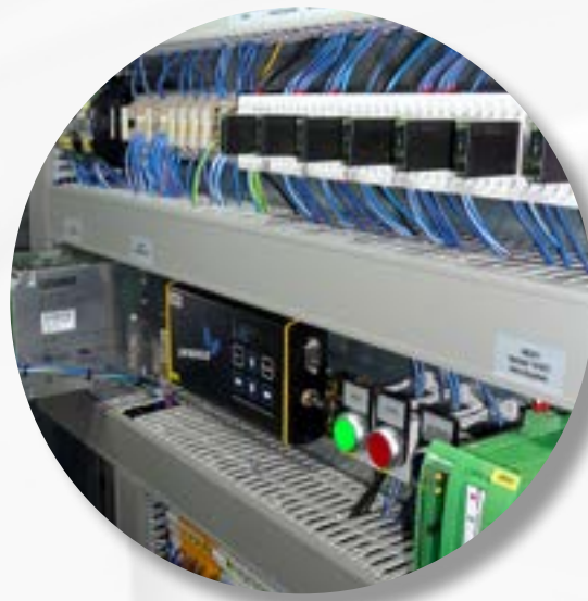
2. Up to now, DATAEAGLE 3000 Master in the control cabinet has been communicating reliably with the cabin.
